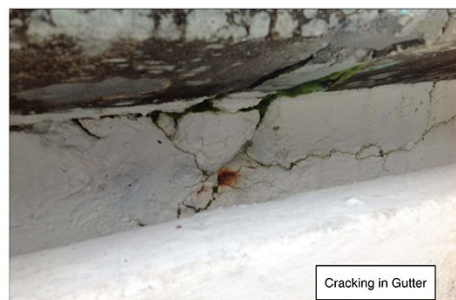
Cracking at Concrete Joint
