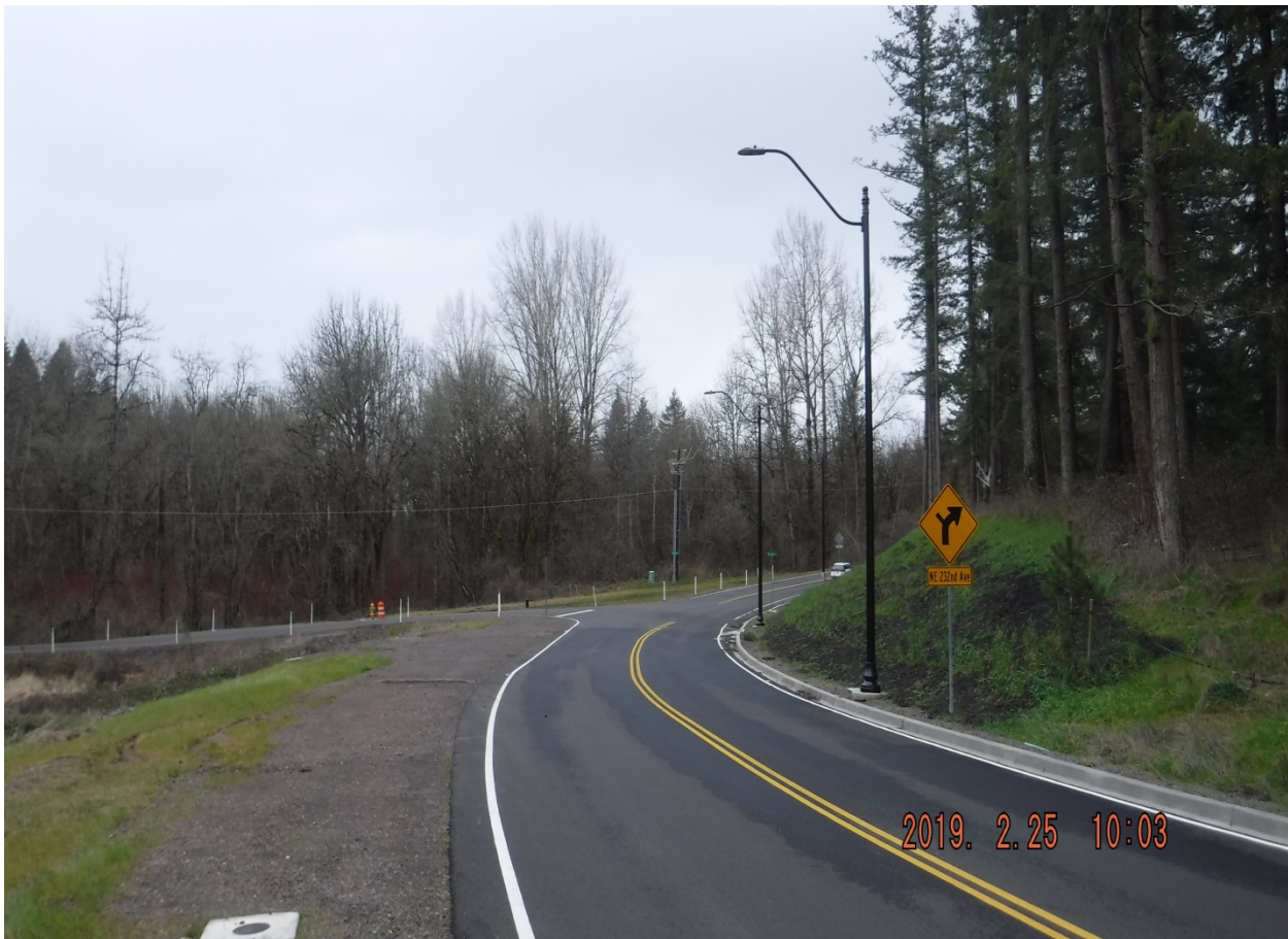
Camas School District Frontage Improvements on North Shore Blvd. (looking north east)
